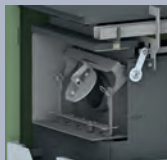
Flue gas flap open
