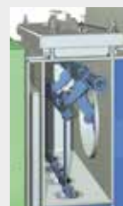
Flue gas flap closed
